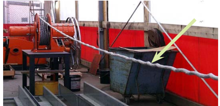
Standard "SO" cable nearing failure at the Gleason Reel Facility
